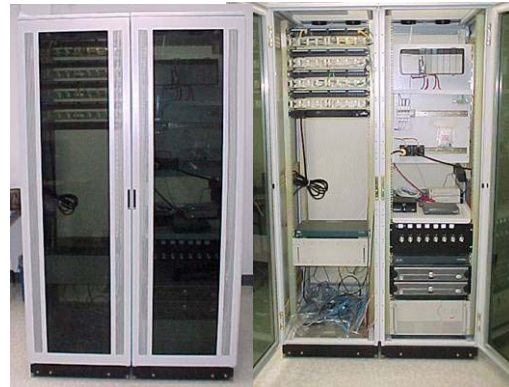
Figure 3 - UtiliData™ Master Station
